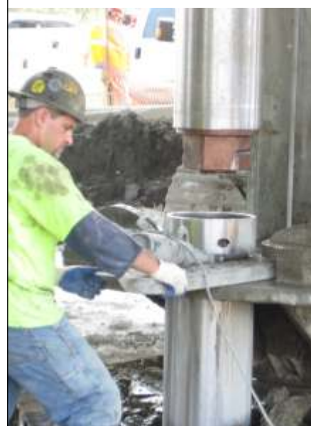
Holte RC Hex Pipe at the White Stone Bridge in New York
